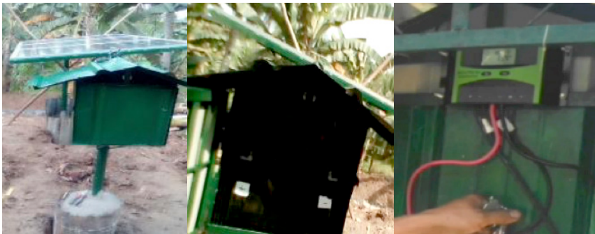
Figure 5. Solar Battery and Charge Controller
